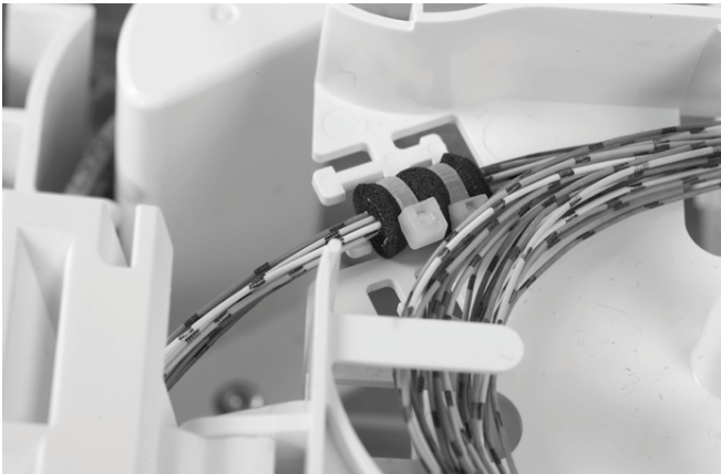
5.10 In case of pre-connectorized MINI PICO cable, fibers are also routed behind the tower and secured with foam and tie-wraps onto the tray.
