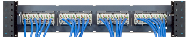
Figure 5 Cabling Modules from the Rear of the Panel
